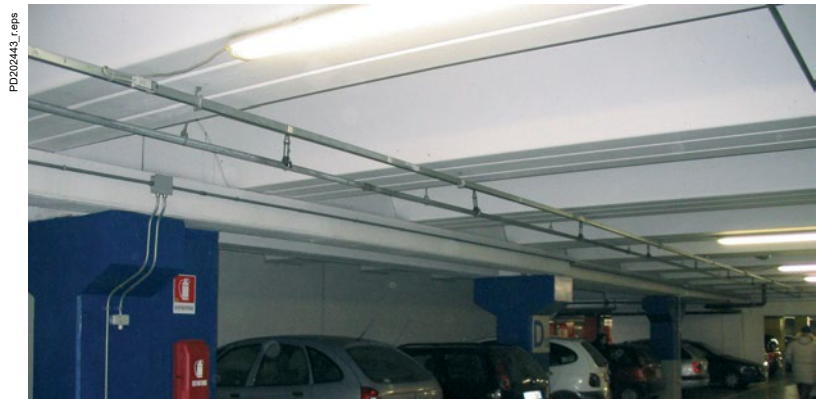
Canalis KBA supplying luminaires nearby sprinklers.
